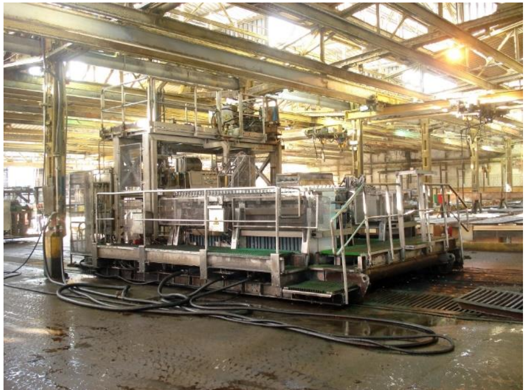
Picture 14. F Cathode Stripping Machine
