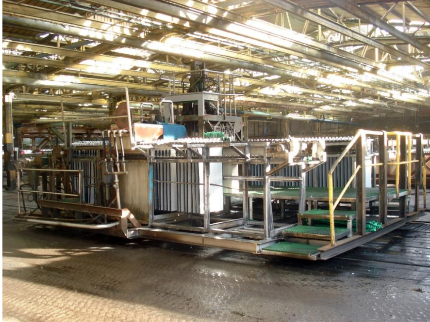
Picture 4. Cellhouse A Stripping Machine
